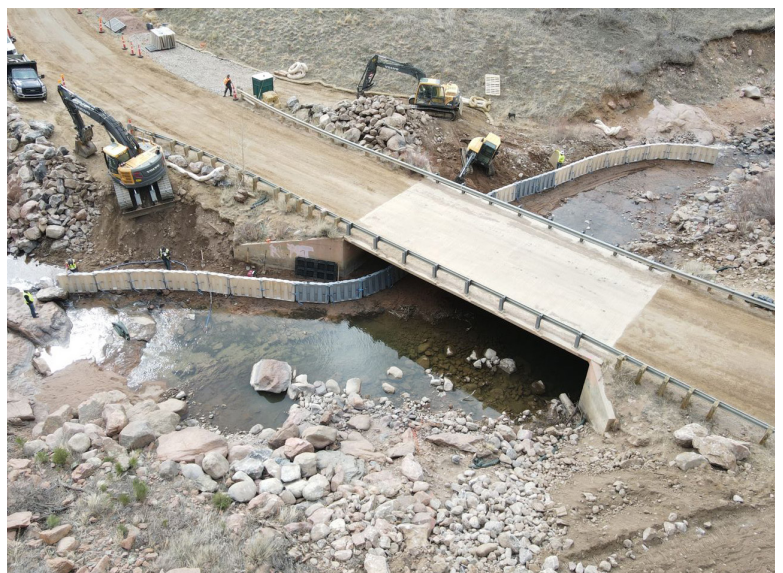
Muscle Wall 4' walls set up and filled with water to create stable channel for diversion of the creek water.
