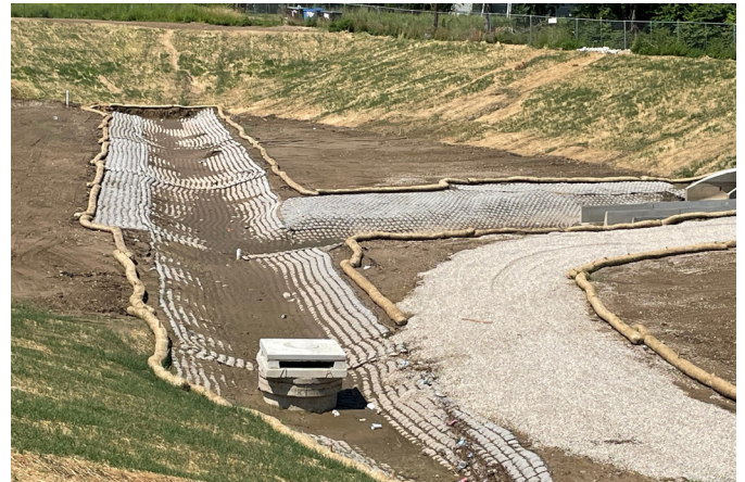
Flexamat installed in the water flow lines to prevent erosion. The site received a lot of rain after installation, so straw wattles are used to keep the mud off the Flexamat.
