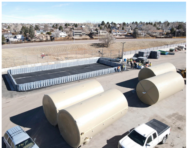
Muscle Wall system set up to form a secondary containment system.
